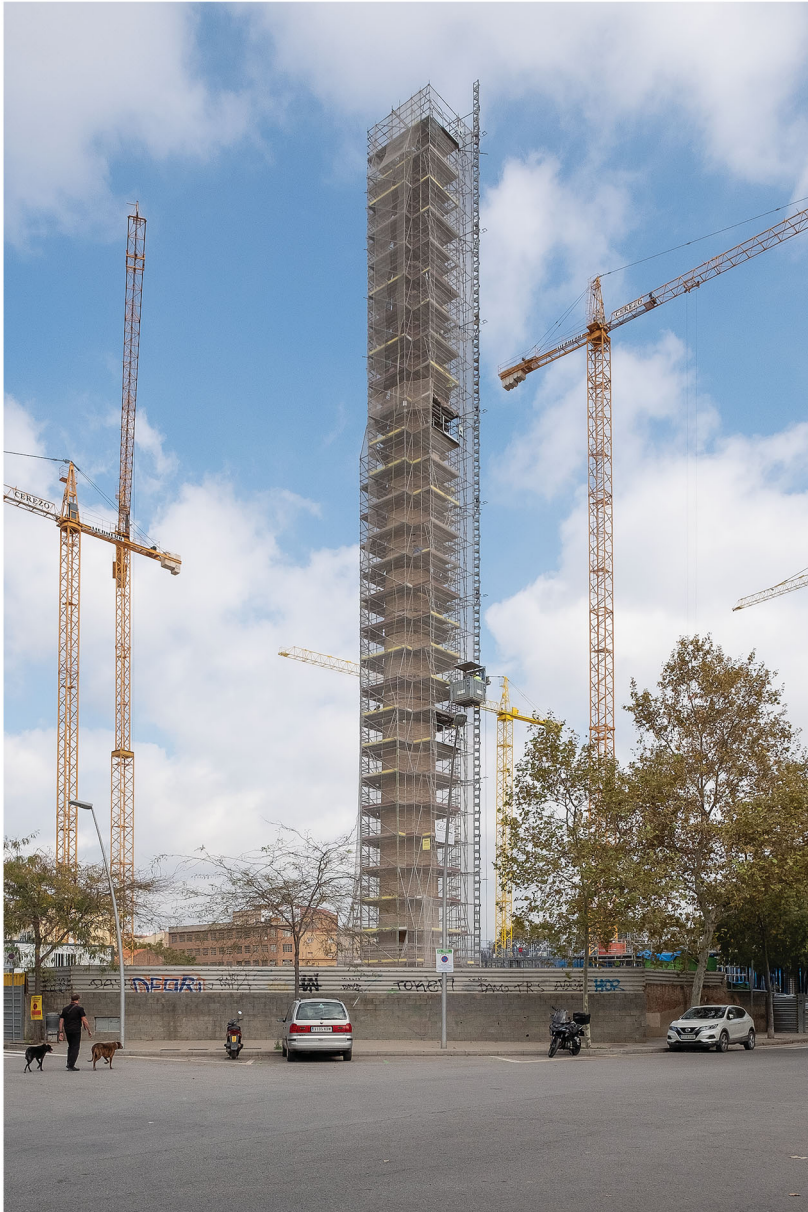
FIGURE 16 The moment of monumentalization: on Carrer de Treball in Poblenou, ensconced in scaffolding, a chimney undergoes structural work. Cranes are poised for large-scale residential redevelopment on the cleared site, 2021.
