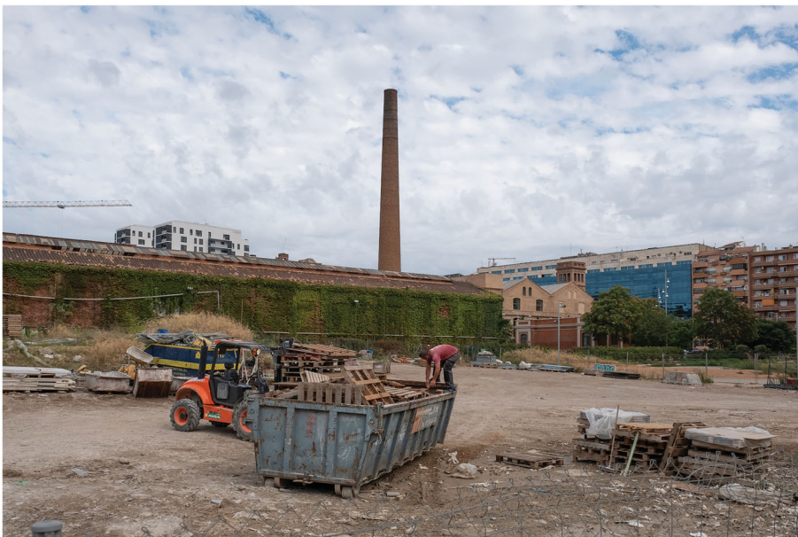
FIGURE 26 Site clearance for the creation of a school and park at the textile mill complex Can Batlló in La Bordeta, 2021.
