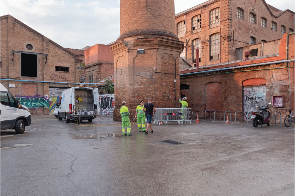
FIGURE 8 Municipal crews remove graffiti from the smokestack of Can Batlló, a massive, partially disused 1870s textile complex in La Bordeta. Since 2011 it has been occupied by a community-run, activist social center. The city is currently converting the site into a park, school, social housing, and the municipal archives, reusing some of the existing buildings. The area around the chimney was converted from parking to a plaza with benches in 2020, 2021.
